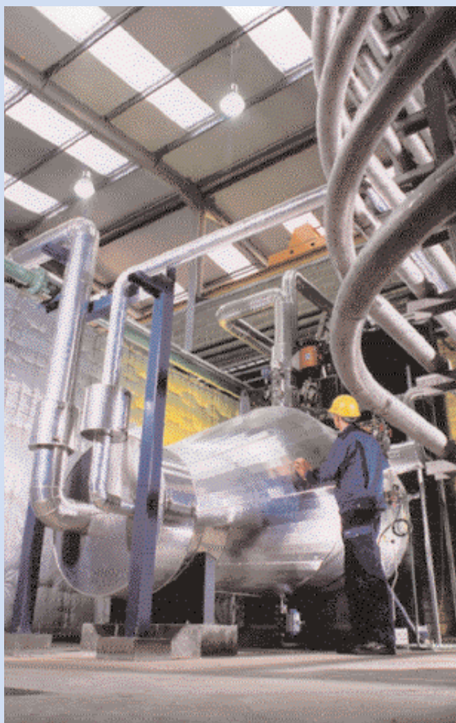
Figure 4: The first commercial scale AquaCat system at Johnson Matthey's Brimdown site in the UK.
